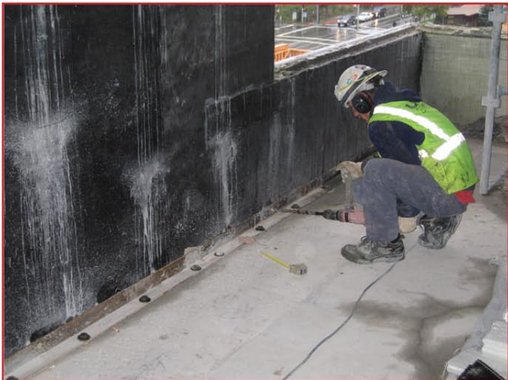
Figure 4: Retrofit of walls with carbon fabric and connection of wall to floor
