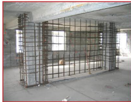
Figure 2: Original retrofit scheme required new shear walls and enlargement of existing columns
